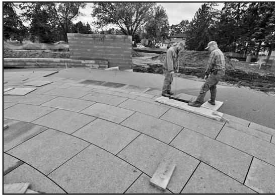
Workers gently placing the granite slabs into their position on the Victory flag plaza. Photo by Randy Klauk.
