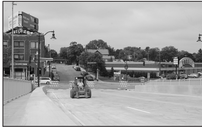
Workers made a last pass before declaring the bridge ready for traffic.
