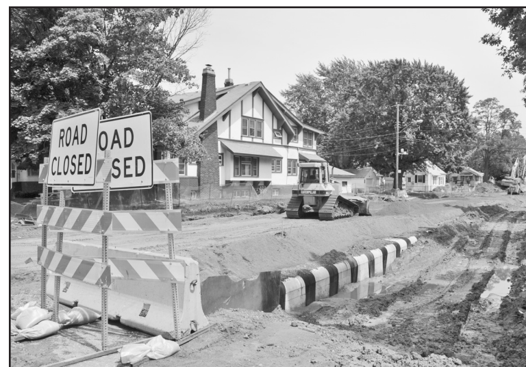
Looking east from Penn Avenue, construction is underway for the 37th Avenue Greenway. Photo by Randy Klauk.
