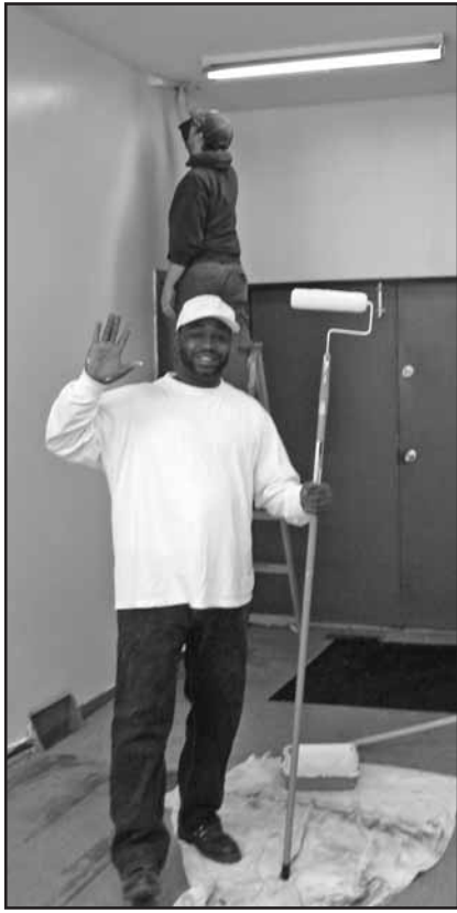
McKinley resident William Bolton waves to the camera while priming the walls of the new McKinley Neighborhood building. McKinley Executive Director Chris Morris is on the ladder.
