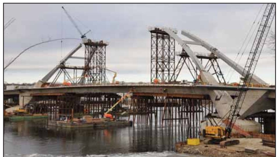
In case you haven't seen the construction lately, here's a view of the new Lowry Bridge (from the eastside looking northwest) taken by Randy Klauk on January 6.
