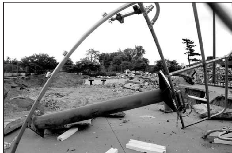
The old pool at Webber Park is being demolished in preparation for a new pool within the next year. Photo by Donna Seline.
